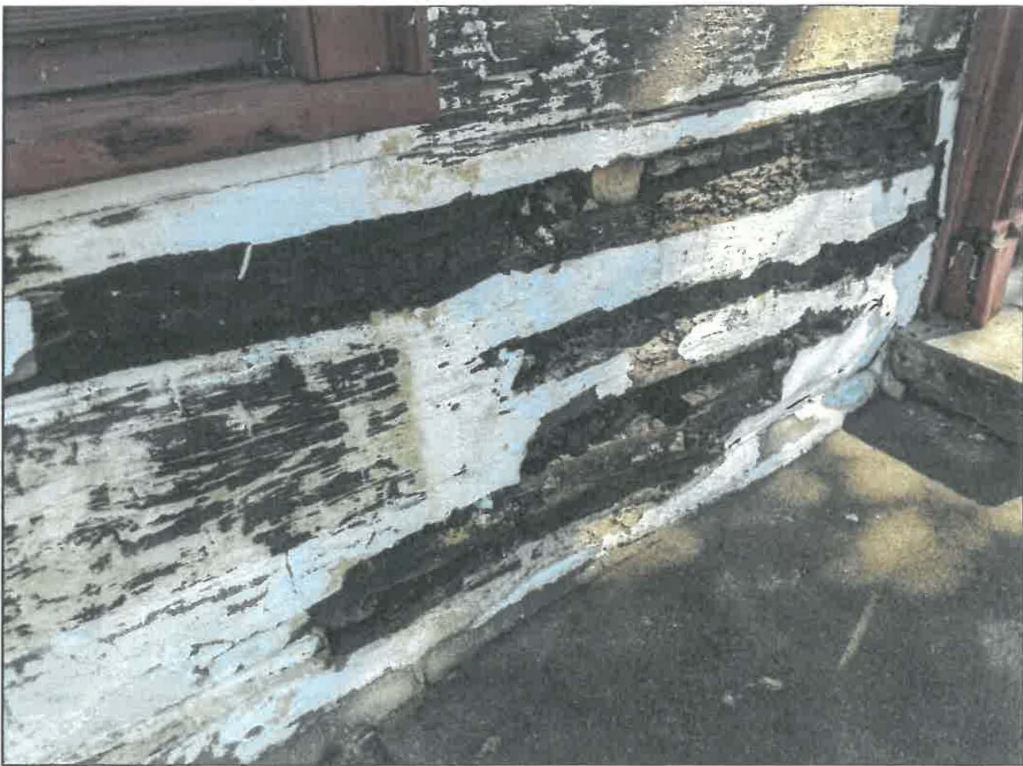
Detail of damage to logs on the south elevation.
