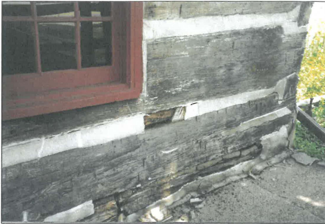
Photograph of the rotten sill log at the southeast corner of the building in 1998 prior to replacement.
