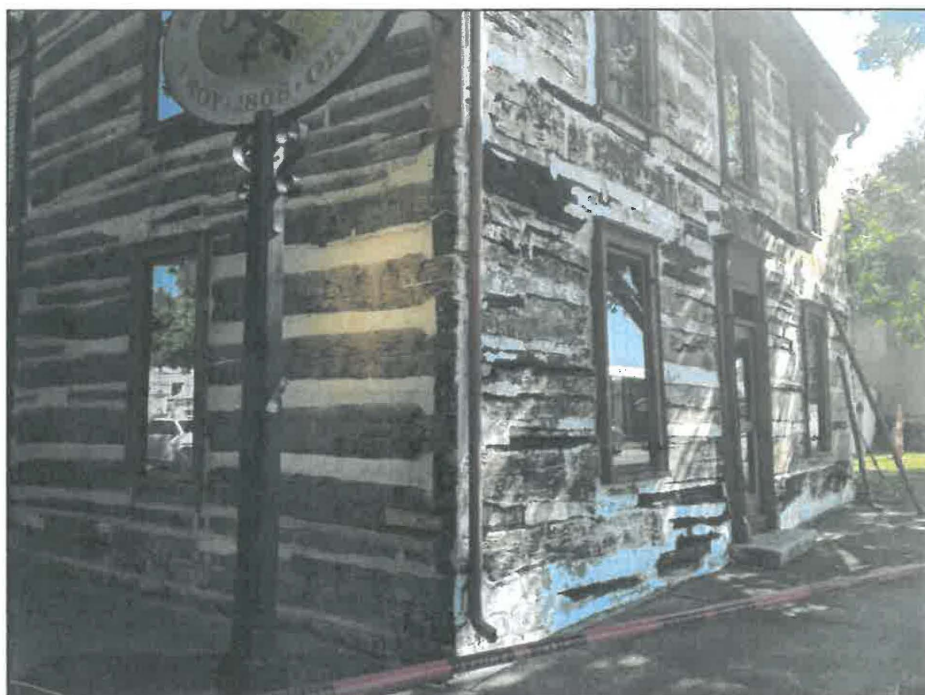
Detail of southwest corner, showing the difference in log preservation between the west elevation, which was protected by wood siding, and the south elevation, which was painted and exposed to the elements.
